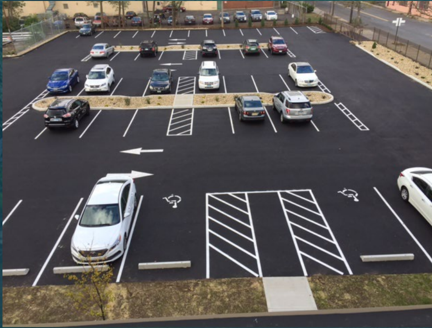
Infiltrating Parking Lot
